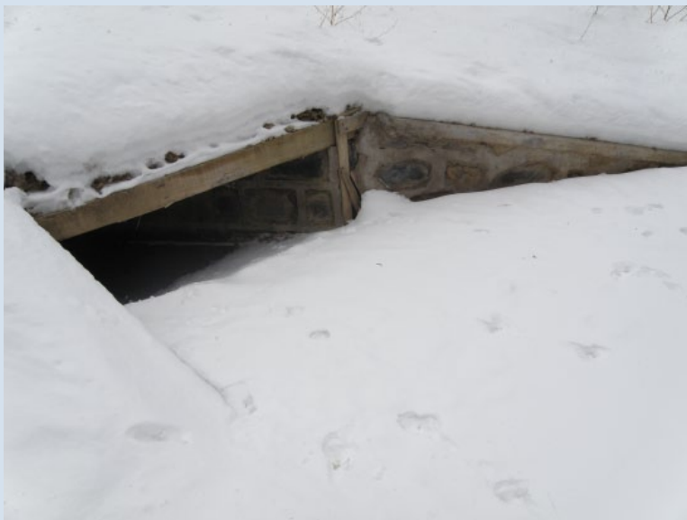
Figure 57.2 Tracks of Siberian weasel through a culvert under the Ring Changbai Mountain Scenic Highway. Source: Photograph by Yun Wang.
